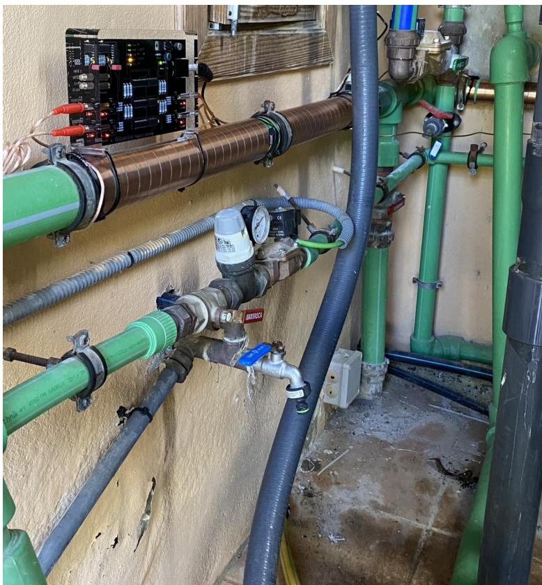
Vulcan S50 in the cold water pipe with Ø 63 mm
